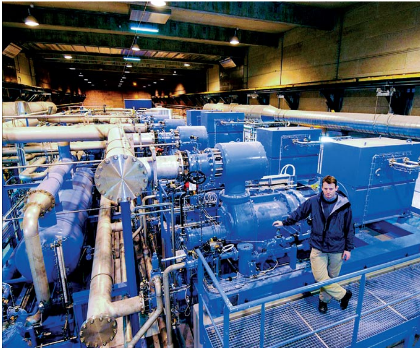
Compressor unit of the 4.5 K refrigerator
